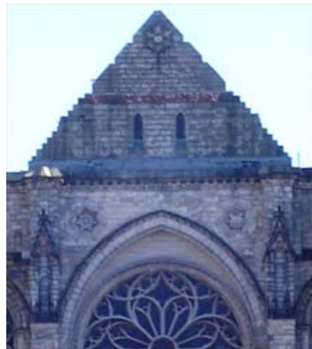
The roof of the Cathedral Church of Saint John the Divine. Home of the REAL environmental movement.
